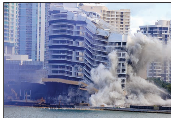
The Mandarin Oriental, Miami was demolished on April 12. Photo courtesy of Alain Martinez
